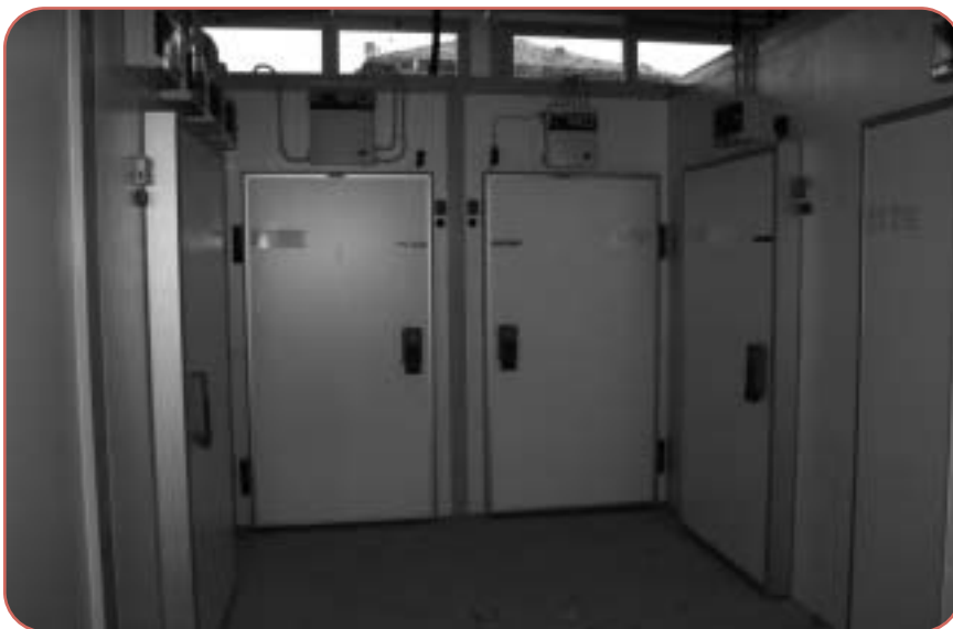
Celle frigorifere - area magazzini/depositi
